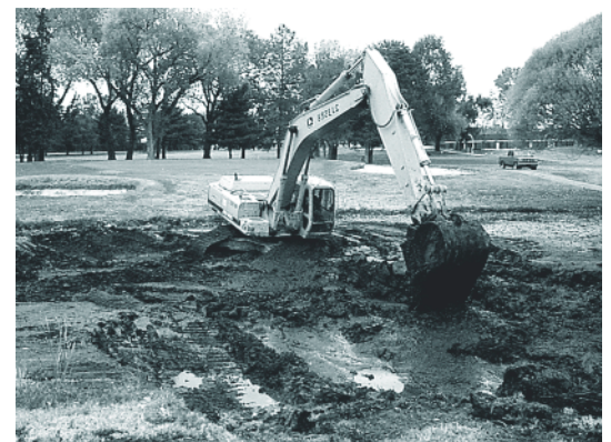
A backhoe removed accumulated sediment from the pond in an effort to improve aquatic habitat and control future algae blooms.
