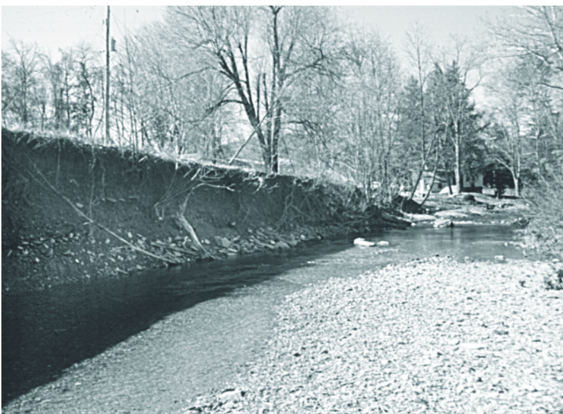
The streambank at the McDannel site was severely eroded at the beginning of the project in February 1999.
