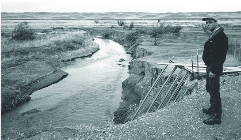
Severe bank cutting and loss of fencing were common on Careless Creek before streambank restoration.
