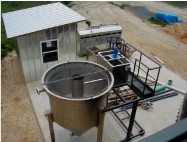
Figure 5. Phosphorus Removal Module at Goshen Ridge Farm
