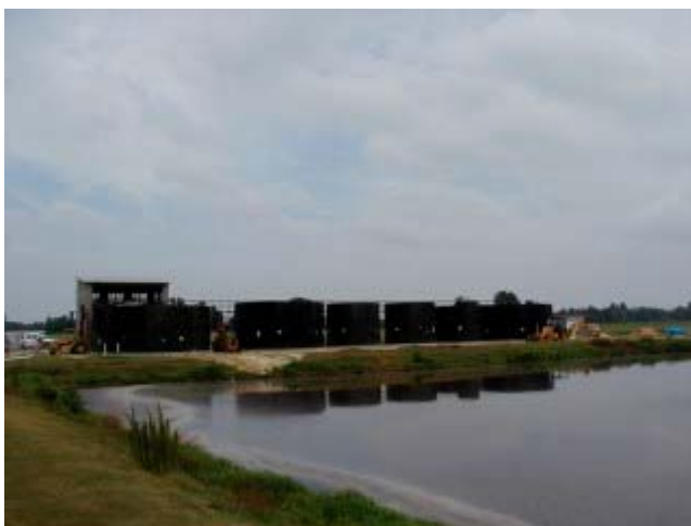
Figure 3. Treatment tanks at Goshen Ridge Farm. First at left is Homogenization tank, last is Treated Water tank, and tanks in between comprise the N treatment process.
