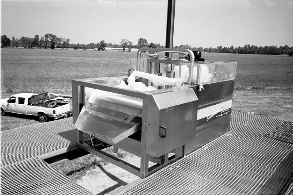
Figure 21. Solid / Liquid Separation Unit
