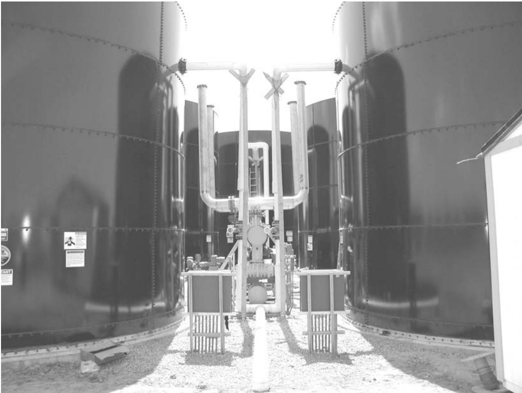
Figure 16. Filter Gallery and Aeration Equipment
