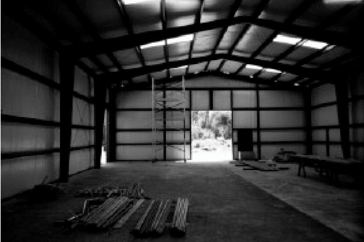
Figure 21. Interior of Solids Processing Facility
