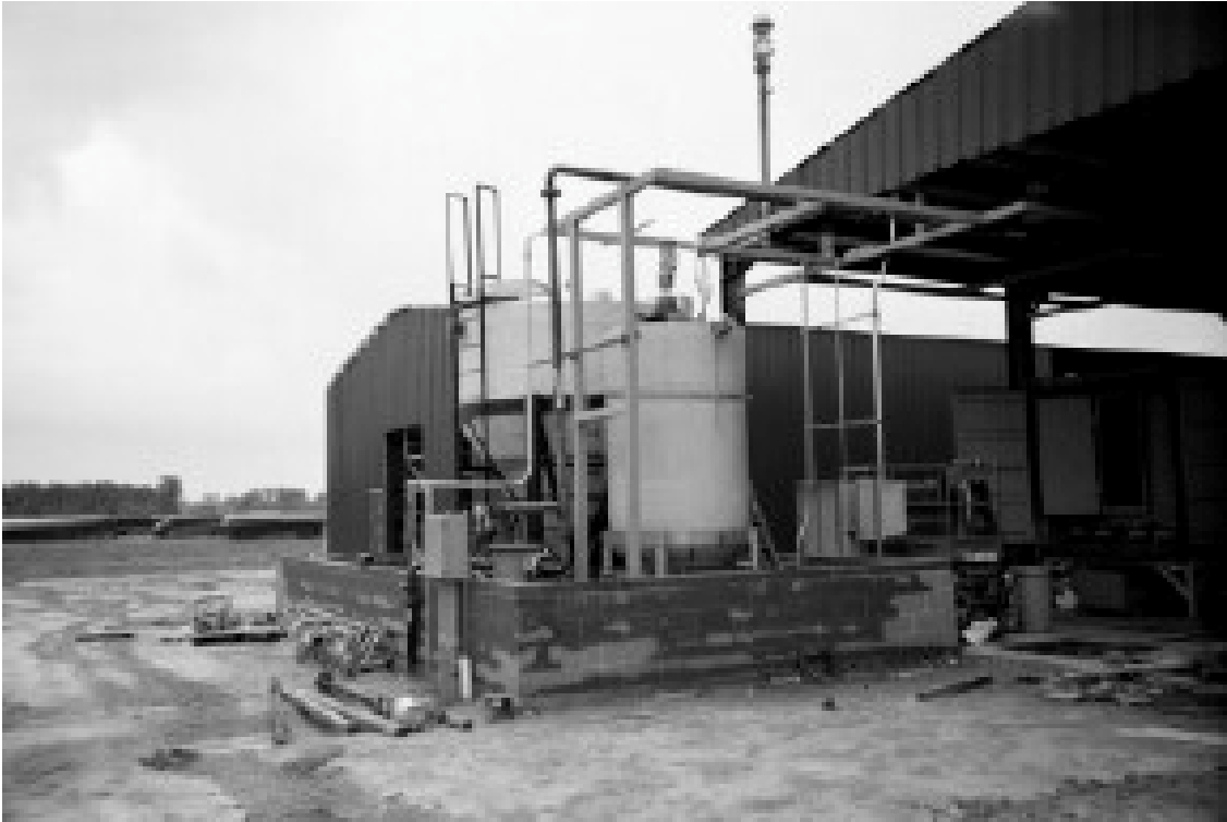
Figure 29. Liquid Pressate Storage
