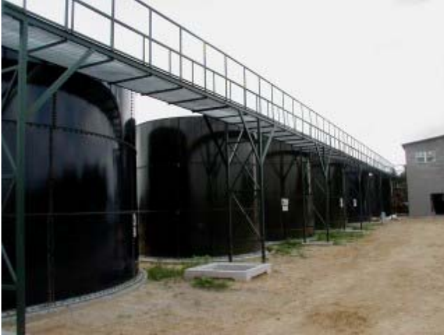
Figure 4. Observation and maintenance platform and N removal tanks at Goshen Ridge
