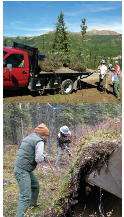
Trail crew members removed mats of vegetation and individual plants from areas slated for construction and utilized these materials to revegetate the disturbed areas.
