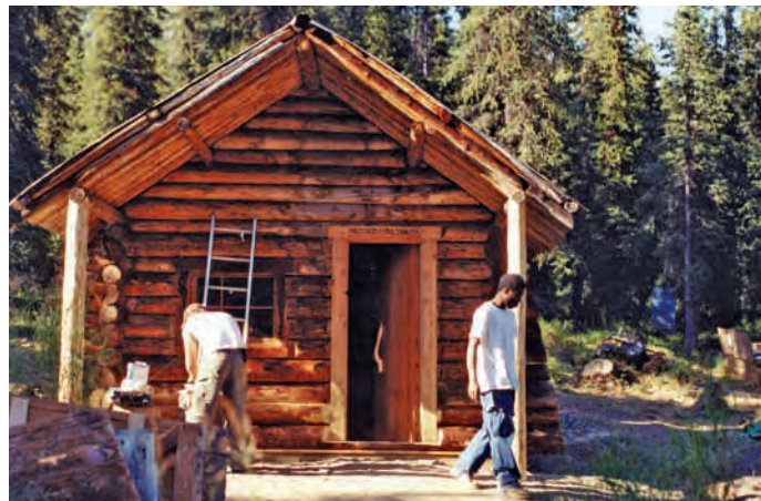
Projects to restore historic cabins, such as the Riley Creek Cabin, are required to comply with the National Historic Preservation Act.
