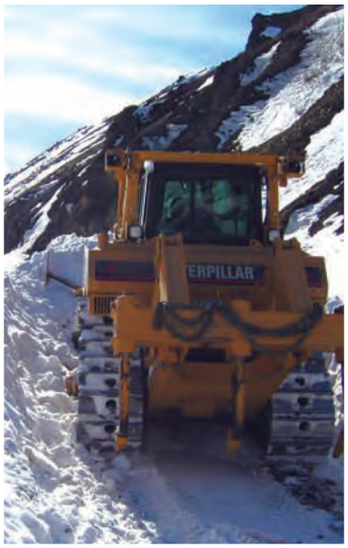
The D7 bulldozer pioneers the first pass up Tattler Grade. It takes more than 11 weeks each spring to clear the 92-mile park road for the operating season.
