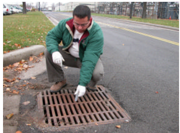
Senior Vector Control Investigator Guy Thomas applying Altosid XR ingot to Storm Receiver Catch Basin
