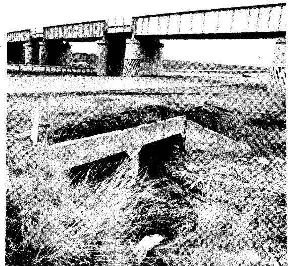
Figure VI-15--Sediment deposition in culvert.
