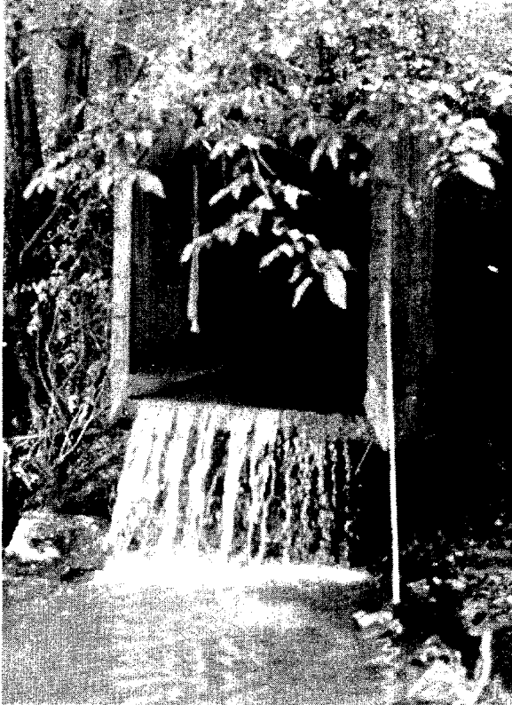
Figure VI-13--Stream degradation at culvert outlet.
