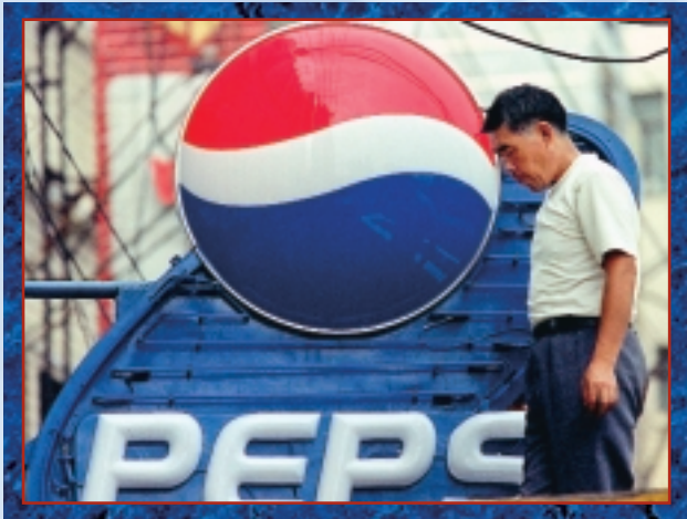
A worker installs a neon sign in downtown Shanghai on October 9, 2000, as key Chinese officials meet to discuss economic development. China entered the WTO in November 2001. AFP Photo/ Liu Jin.
