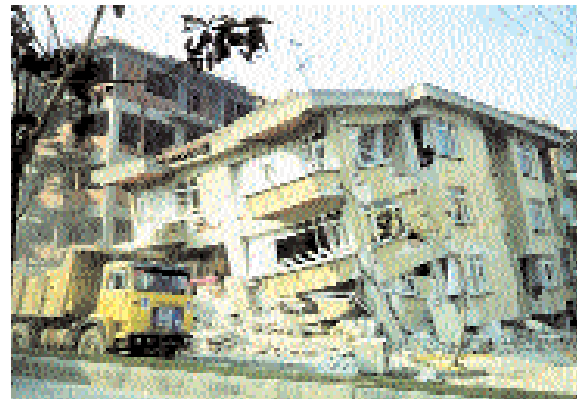
Damage caused by the 12 November earthquake. Duze, Turkey
