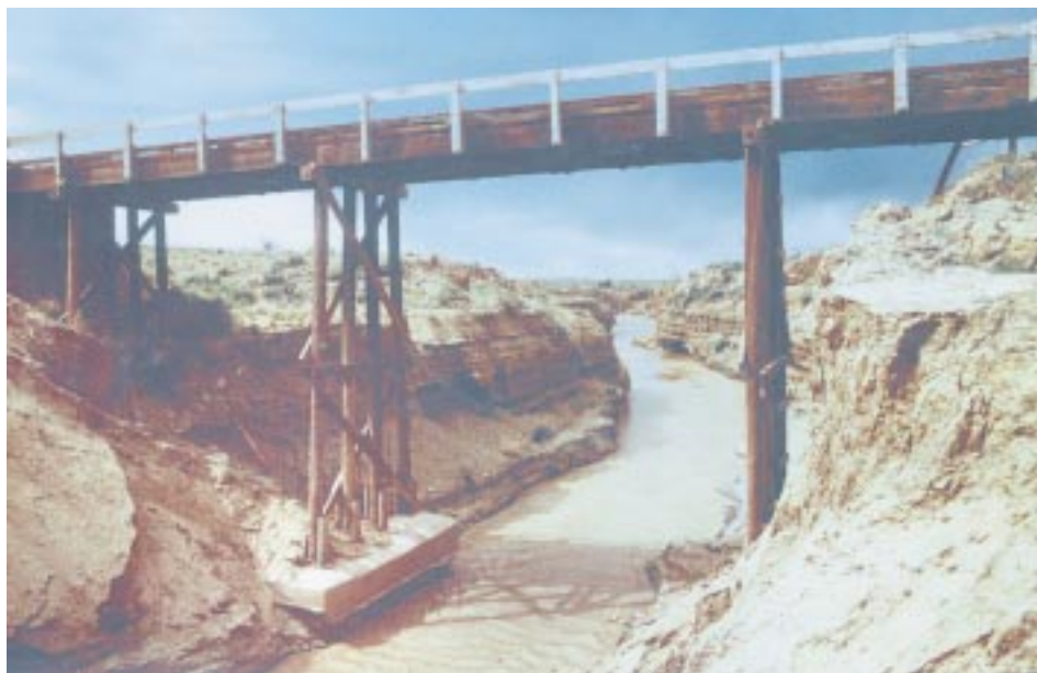
Bridge scour on Rio Puerco River, New Mexico. Photo courtesy of Steven D. Craigg, U.S. Geological Survey.
