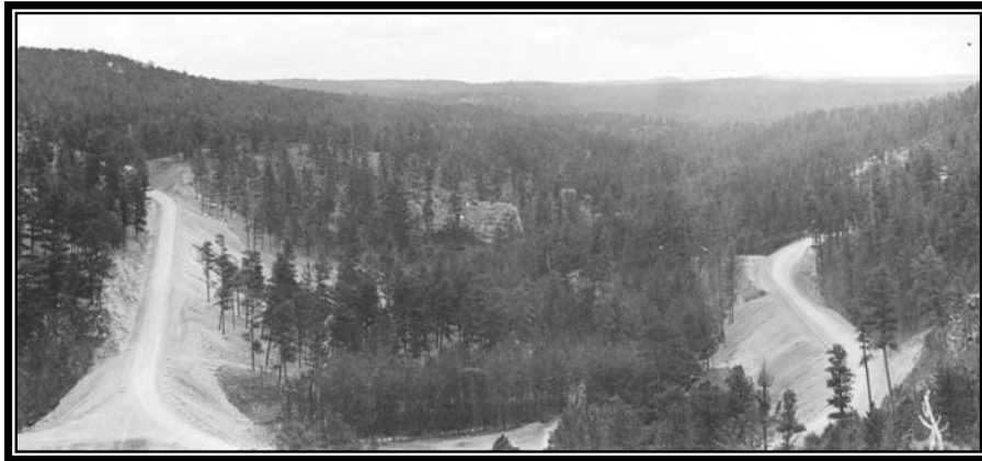
Figure 7-3. Construction of the new road that passed the Jewel Cave National Monument cave opening, completed in the mid-1930s. Courtesy of the Mount Rushmore National Memorial (JECA 2896).
