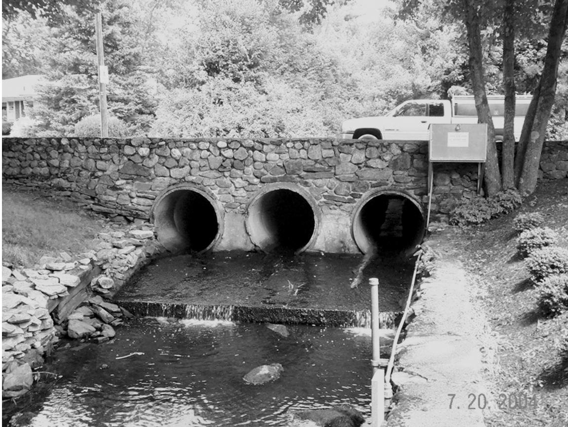
Culvert pipes at USGS streamflow gaging station (instrument shelter at right) on Catamint Brook at Cumberland, RI, 01113685.
