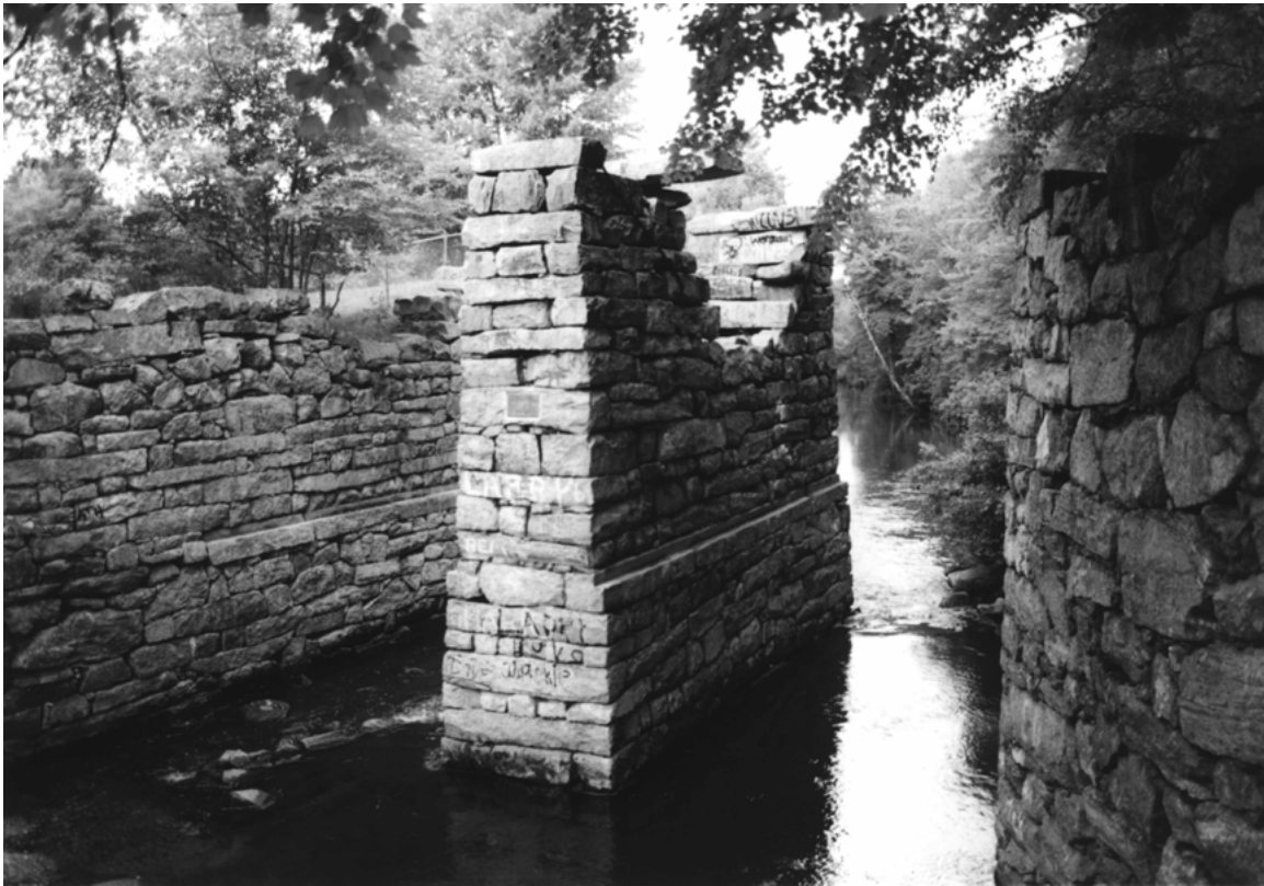
Remains of support piling for the Middlesex Canal (National Historic Landmark), operated from about 1793 to 1853, Shawsheen River, Wilmington, Mass. (photo by R. S. Socolow).
