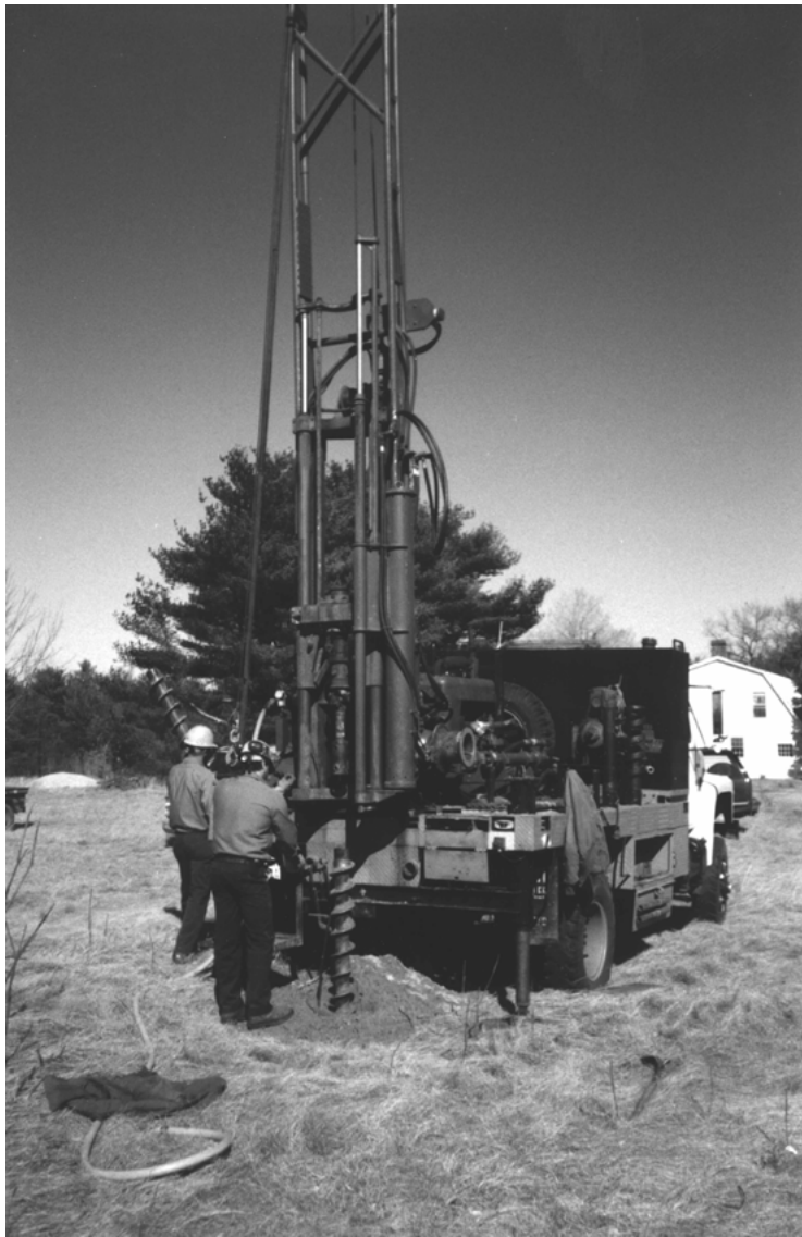
USGS drill rig installs ground-water-level observation well, Princeton 64, in Princeton, Mass. (photo by R. S. Socolow).
