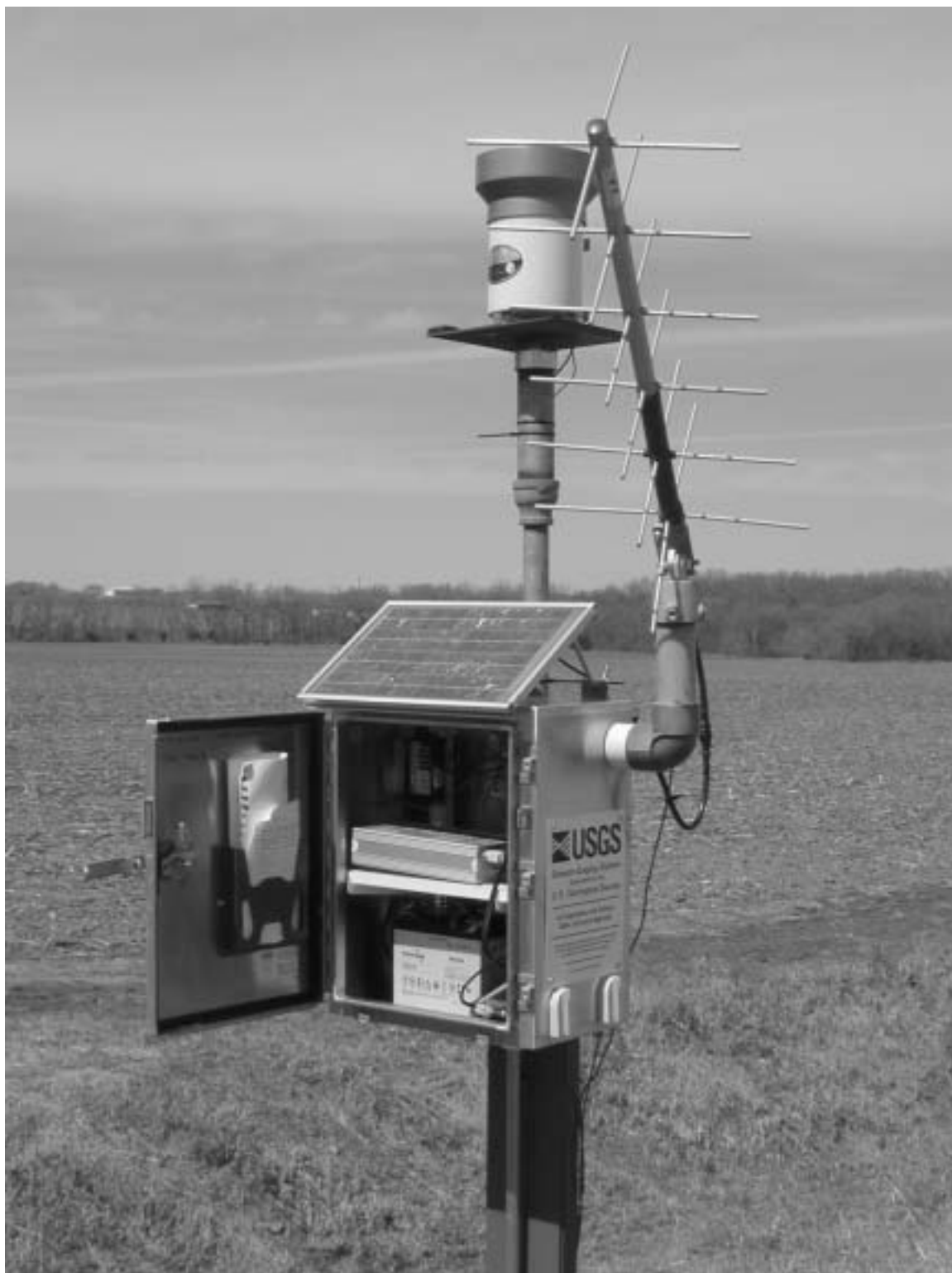
New streamflow-gaging station established on Wakarusa River near Richland (station 06891260), October 25, 2002. Photograph courtesy of J.R. Barnard.
