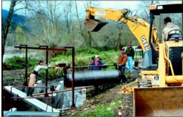
Figure 2—Applegate Watershed Council crews work to install a “fish-friendly” intake pipe for irrigation on private land. Photo by Jan Perttu
