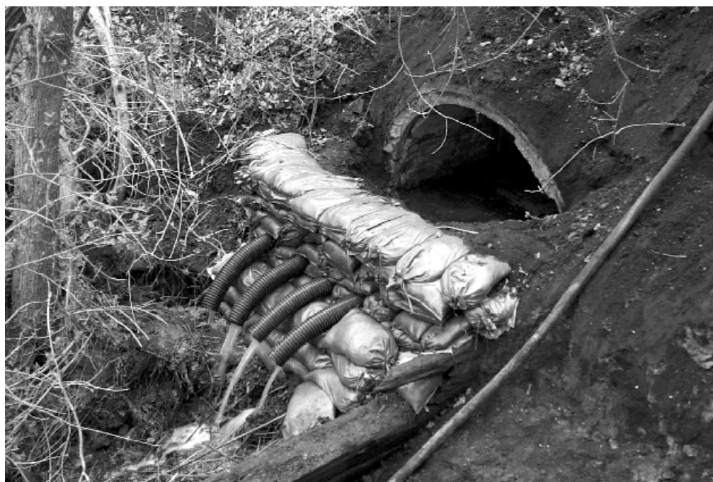
An underflow dam in a drainage culvert blocked the flowing oil.
