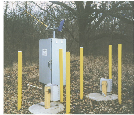
Multiple Sensor data-collection platform (DCP) installation in Kansas.
