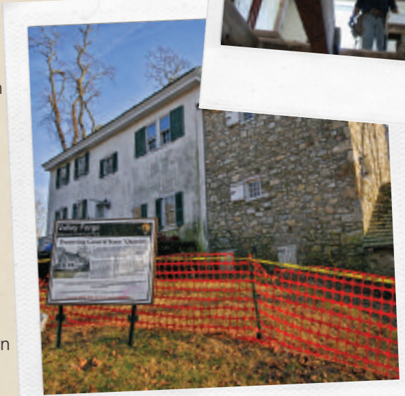
Rehabilitation after two centuries of wear and tear on General Henry Knox' Quarters included major structural repairs and a new roof.
