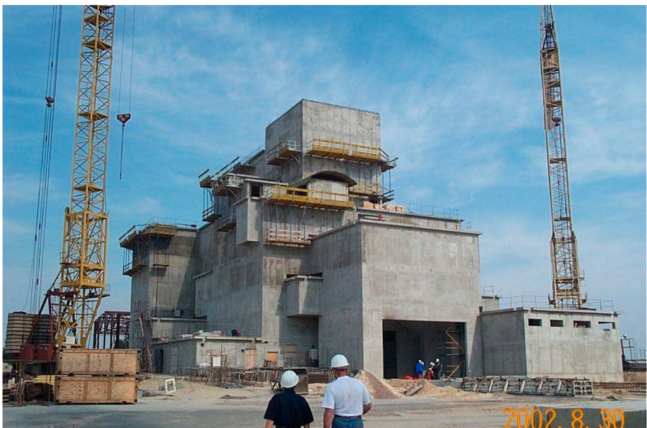
▲ Spent Fuel Conditioning Facility
