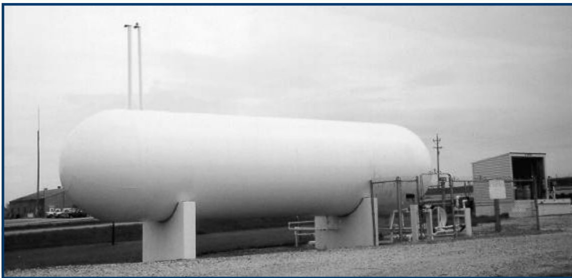
An 18,000-gallon propane tank with protective fencing to reduce the risk of physical damage to the exterior piping system.
