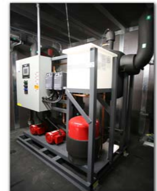
SNPS Medium Temp Pump Stations
