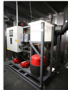
SNPS Medium Temp Pump Stations
