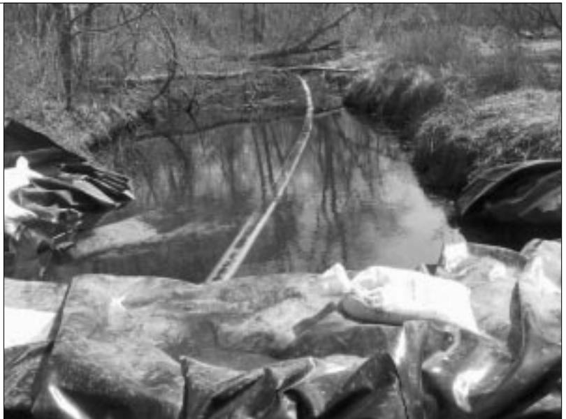
A temporary dam and diversion pipe helped dry a portion of the river where vacuum guzzling was tested.
