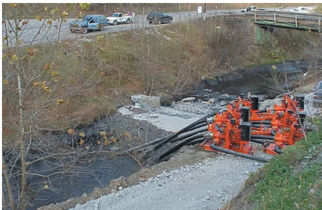
Figure 3 Mobile pumping stations extend the unit's pumping range.
