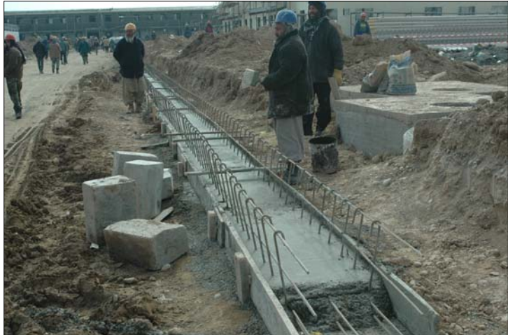
Afghan workers place concrete for the curb and drainage system that will run throughout the ANCOP compound in Lashkar Gah. [USACE Photo]
