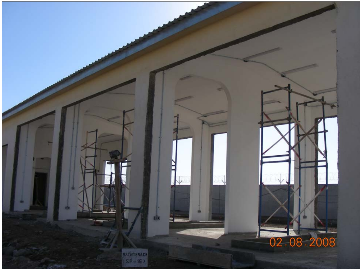
A large vehicle maintenance facility which is equipped with underground maintenance bays is painted before contractors install the large overhead doors. [USACE Photo]
