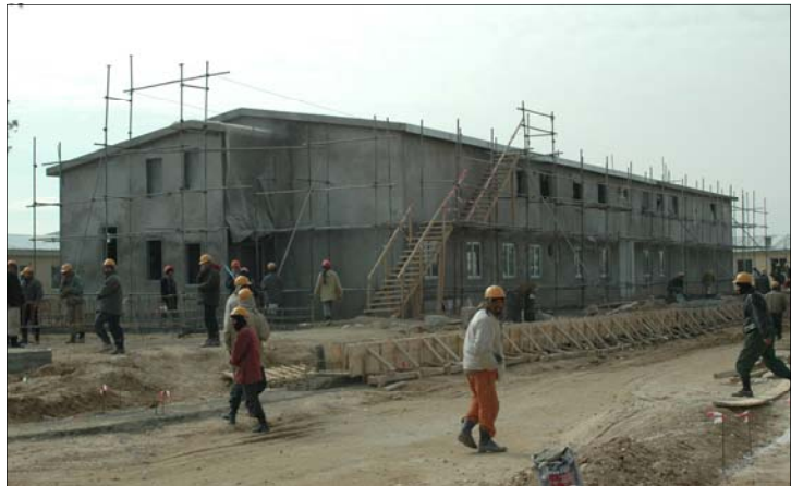
Afghan workers put the finishing touches on a two-story barracks at the ANCOP compound. [USACE Photo]
