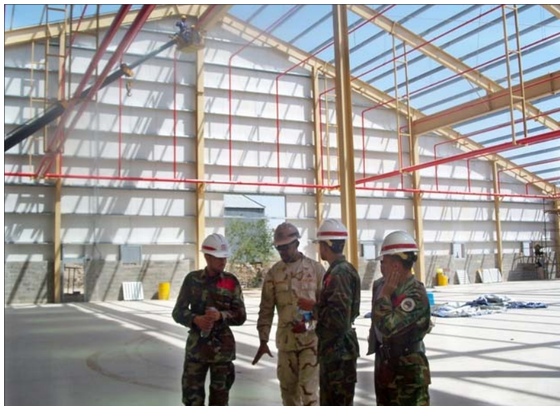
Construction Representative William D. Breckinridge (2nd from left) discusses with the Cadets how the foundation and concrete slab was constructed at a logistics warehouse and how long it took. (Photo by Leslie J. Wright, Capacity Development Program Manager)
