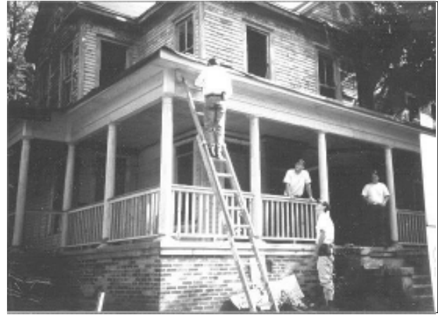
Contractors rehabilitate an older building for use as affordable housing in Macon, Georgia. (Photo courtesy of the National Trust for Historic Preservation)
