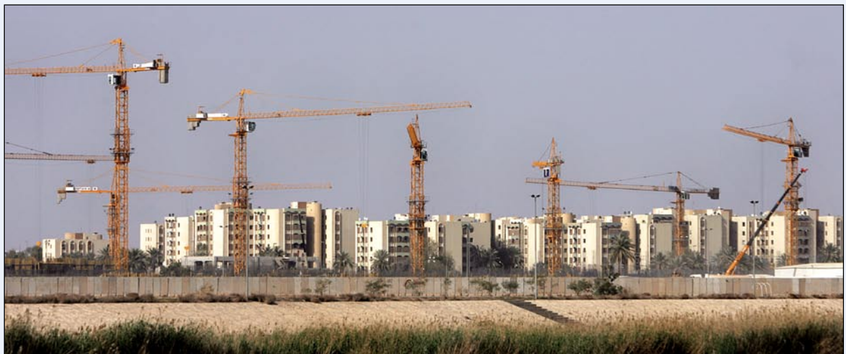
Construction cranes tower above the building site of the U.S. embassy in Baghdad, Iraq, March 2006. AP/Wide World
