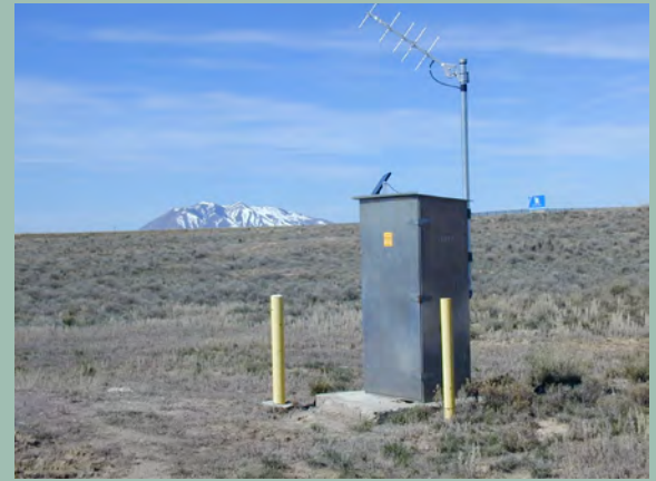
Real-time monitoring well that is part of the USGS Ground-Water Climate-Response Network in Idaho (photograph by Matthew Gilbert, USGS).
