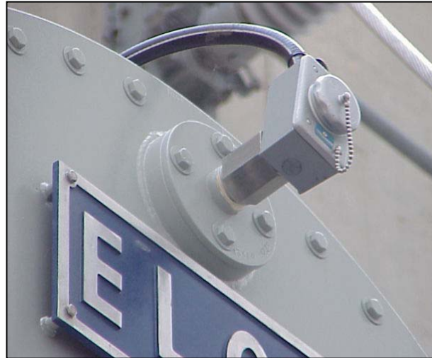
Figure 13.—Bladder Failure Relay.
