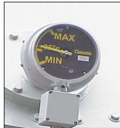
Figure 8.—Conservator Oil Level.
