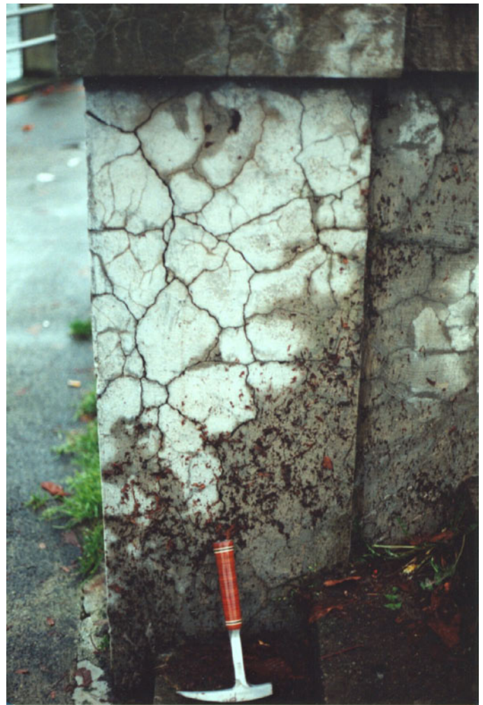
Figure 2. Concrete column in Stanley Park, Vancouver, British Columbia, showing typical “map” cracking throughout entire column, induced by expansion of concrete due to swelling alkali-silica gel. Reactive aggregates include andesite and dacite from Mount Garibaldi near Whistler, British Columbia, as well as quartzite, chert, and granodiorite. Concrete was cast in the 1920s; specific aggregate source (that is, location of pit) is unknown.
