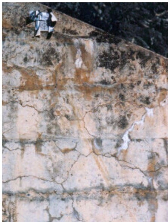
Figure 10. Section of a wall in a dam in southern British Columbia, showing well-developed “map” cracking and efflorescence, both indicators of alkali-silica reaction. Concrete was about 47 years old at time of photograph.
