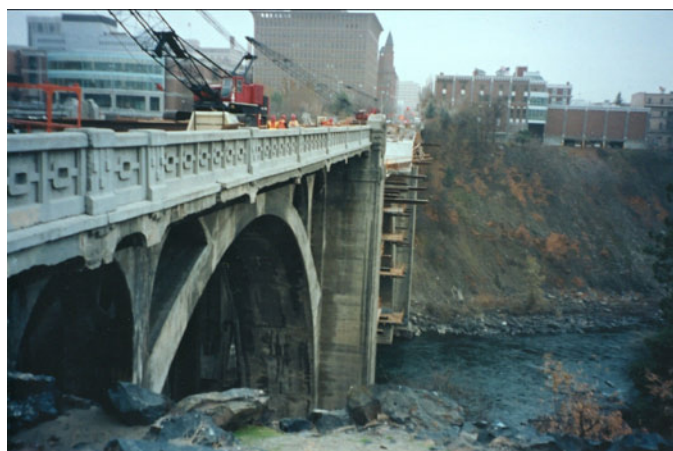
Figure 13. Closeup of Monroe Street Bridge, Spokane, Washington, showing section of main arch. Concrete removed from demolished sections was determined to have been affected by alkali-silica reaction.
