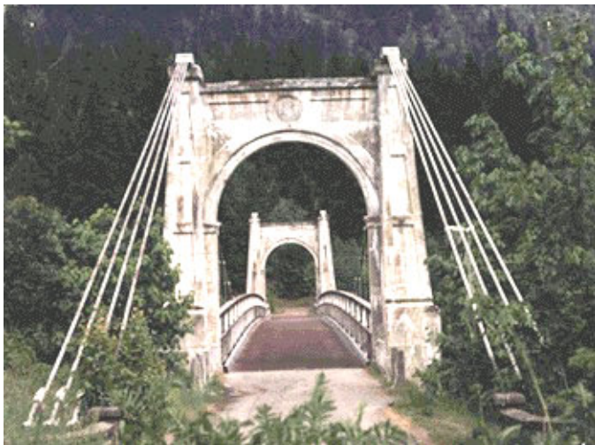
Figure 5. Old Alexandra Bridge in Fraser Canyon, near Boston Bar, British Columbia, showing piers and abutments damaged by both alkali-aggregate reaction and freeze-thaw cycles.
