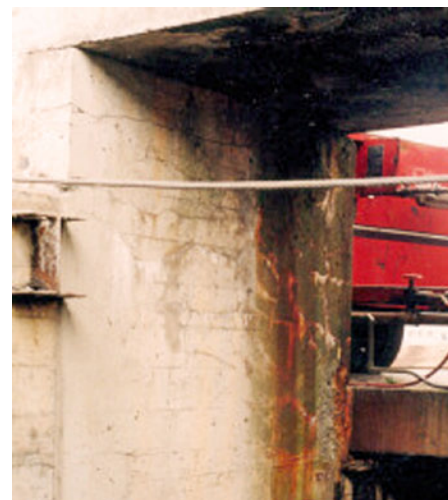
Figure 6. Part of a dock structure in Vancouver, British Columbia, showing “map” cracking. Reactive aggregates include Mount Garibaldi volcanic rocks, opal (in volcanic vugs), granitic rocks, and quartzite. Aggregate was derived from the now-closed Britannia Pit, located near Squamish, British Columbia.
