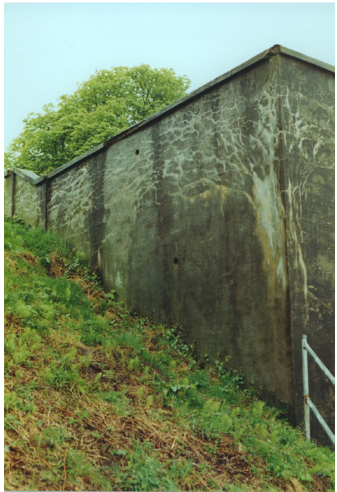
Figure 4. Wall in Stanley Park, Vancouver, British Columbia, showing white deposits of leachate emanating from cracks in concrete. These “efflorescence” deposits are composed of a mixture of alkali-silica gel and calcium carbonate.
