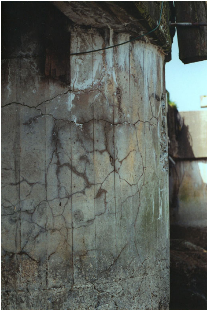
Figure 3. Pier in Seattle harbor, showing well-defined “map” cracking induced by alkali-aggregate reaction. Reactive aggregates include andesite from the Mount Rainier-Mount St. Helen’s area, Wash., as well as sandstone, chert, and quartzite of unknown provenance. Field of view, 1 by 1.3 m.
