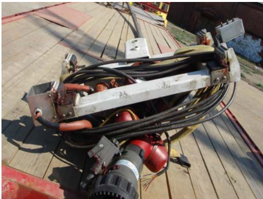
Photo 4 – Monitor and pipe that “launched”
