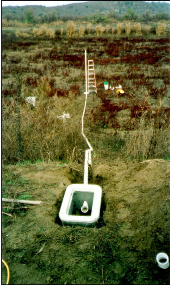
Water Level Recording Equipment and Staff Gage Installation February 15, 2000
