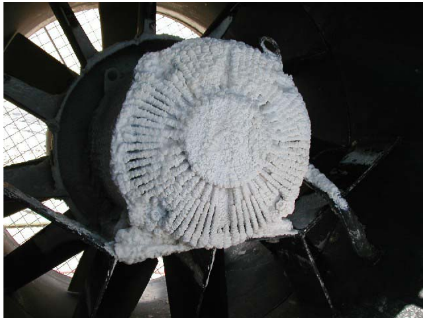
Figure 5.8—Salt deposits on evaporators from mist ingestion.
