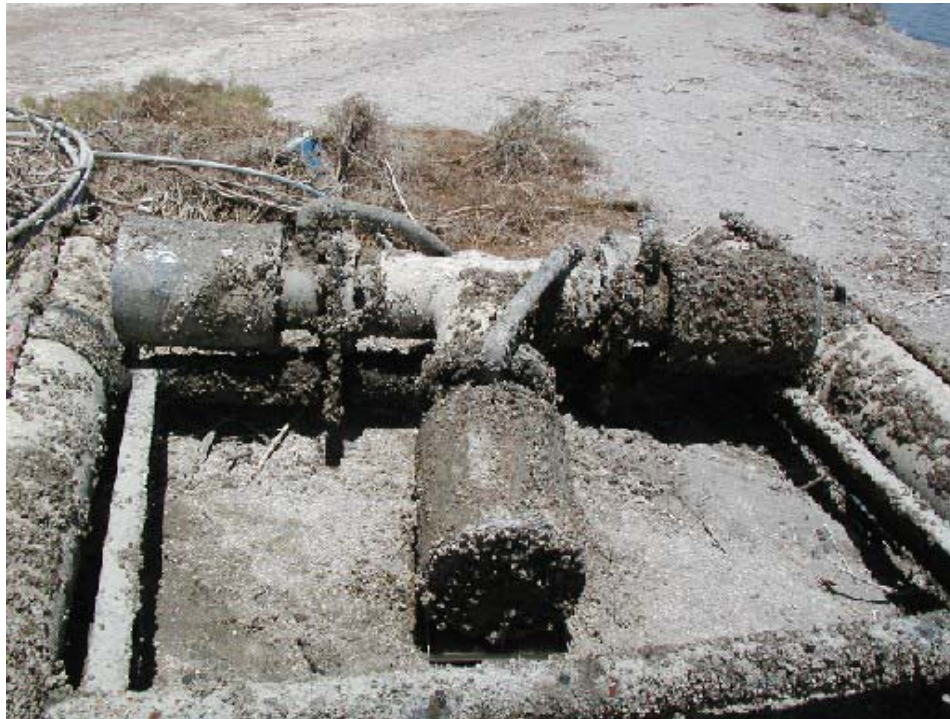
Figure 5.10—Barnacle fouling of intake structure and fish screens at Bombay Beach solar pond facility.
