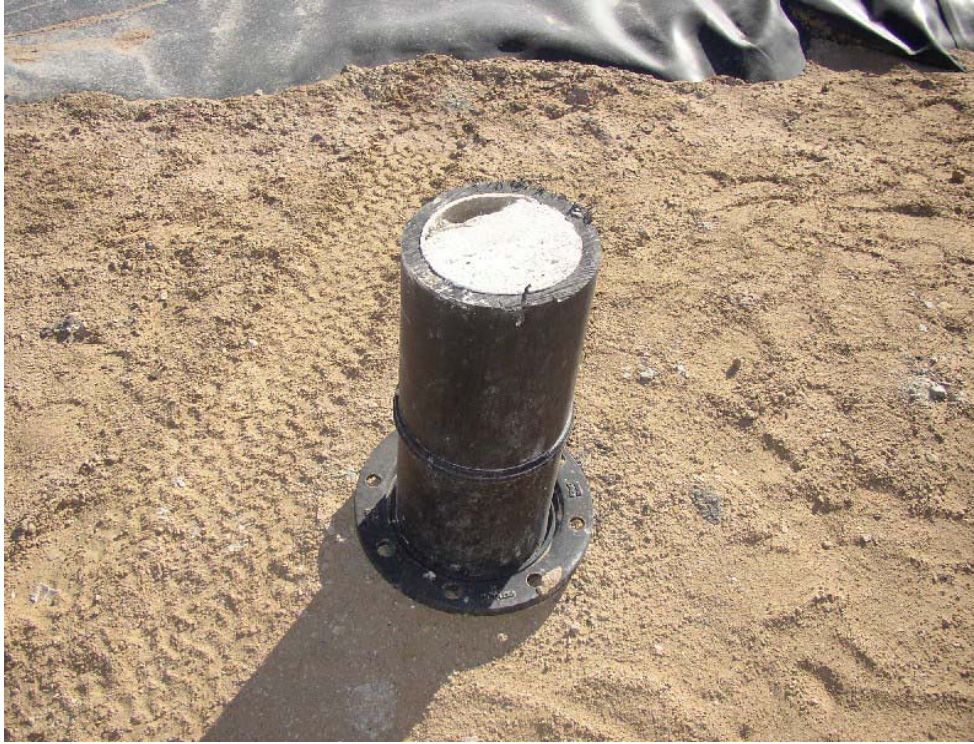
Figure 5.1—Gypsum fouling of closed conduits.
