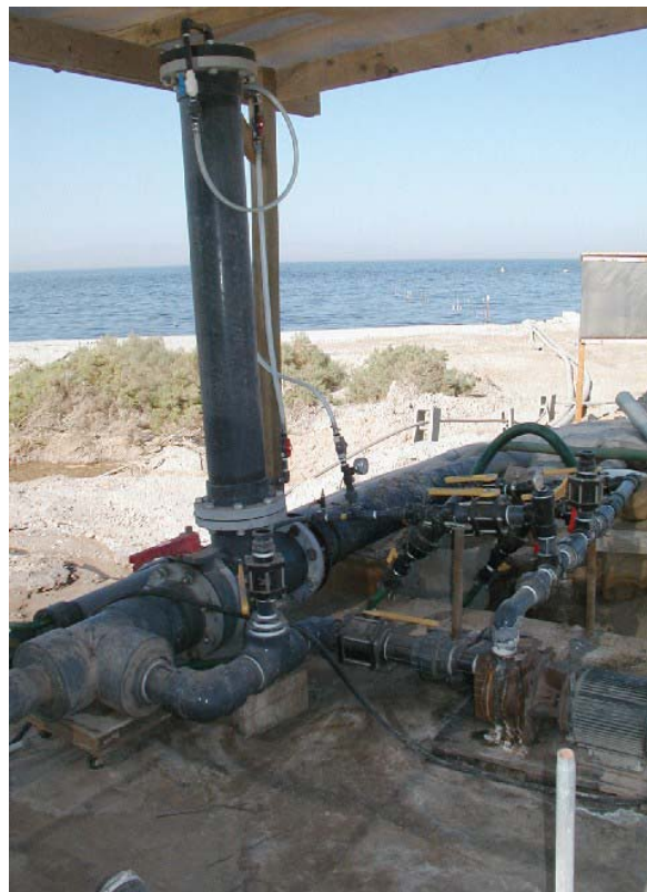
Figure 5.12—Intake structure degassing facility.
