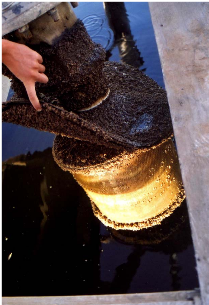
Figure 3.12—Self-cleaning intake screen.
