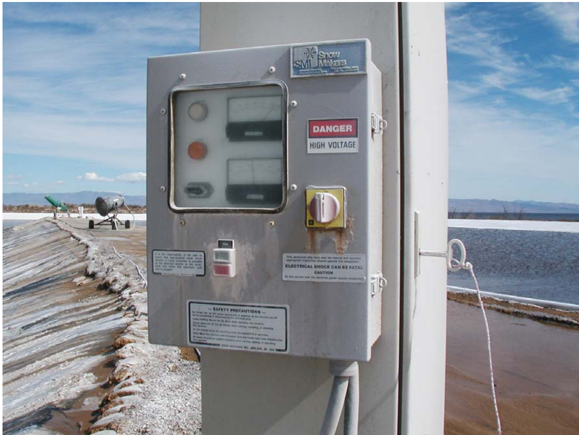
Figure 3.13—Electrical control box for enhanced evaporators.
