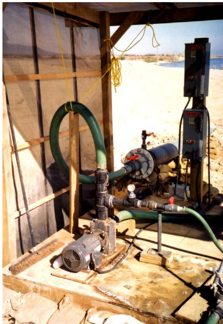
Figure 3.11—Sea intake pump.
