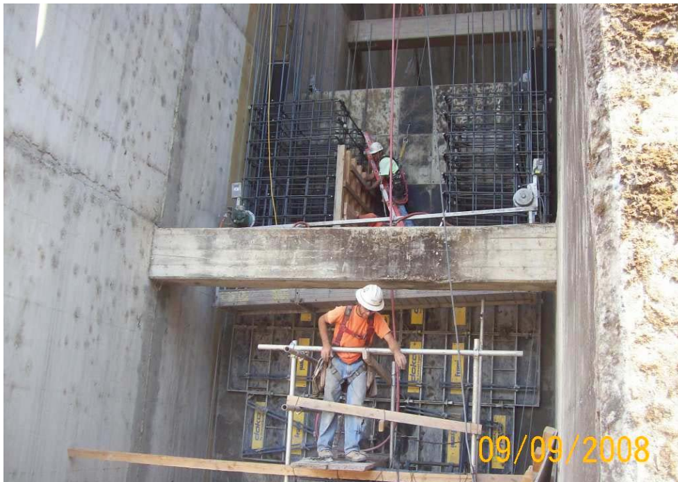
Workers are setting up formwork and installing reinforcement in preparation for a concrete placement in the diaphragm walls on the south side of the dam. Scaffolding is being removed and relocated to the next higher lift placement.
