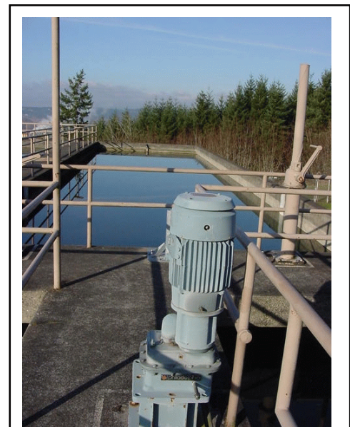
Presedimentation basin with flocculator in foreground.
