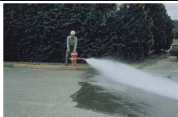
Unidirectional flushing at high velocities can scour water mains, removing corrosion products, biofilm, and sediment.
