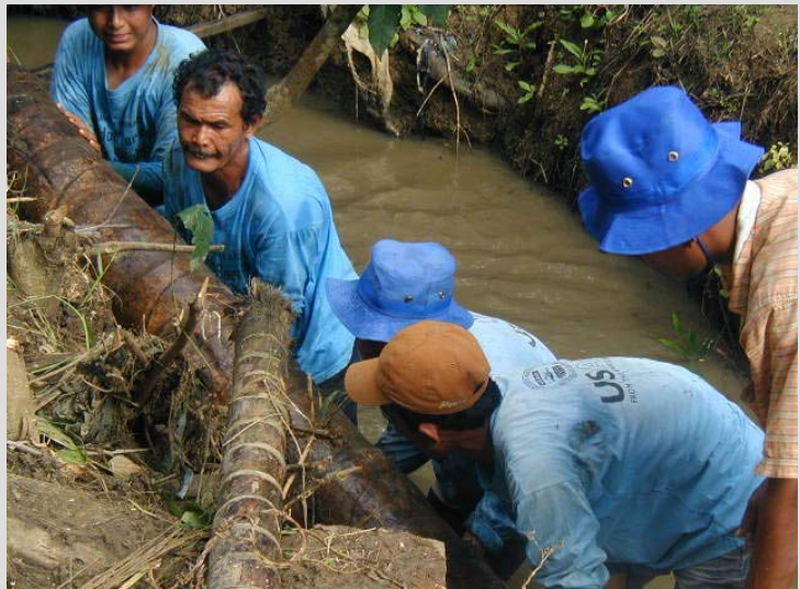
Through a cash-for-work initiative, villagers work to remove fallen trees from the irrigation canal.
