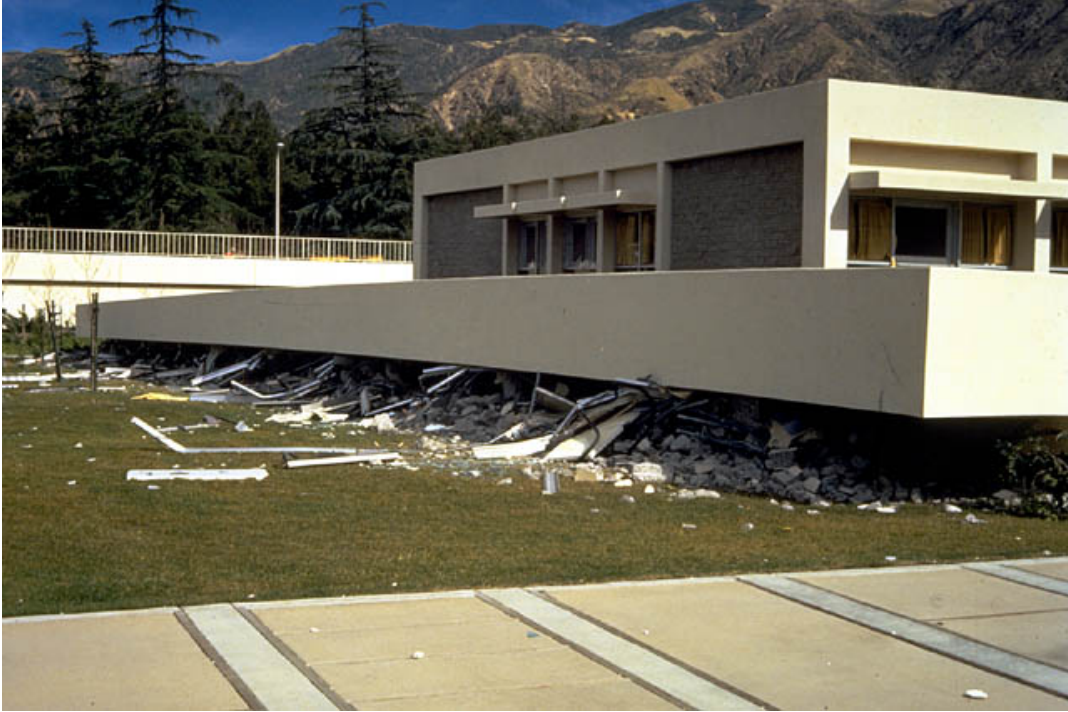
Figure 4-8. Second story of psychiatric unit, Olive View Hospital, 1971, pancaked over first story. This and other damage at Olive View Hospital emphasized the poor seismic performance of NDRC construction.
