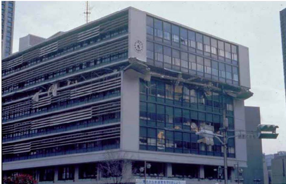
Figure 4-6. Collapsed story of steel moment-frame building, Kobe, Japan, 1995.
