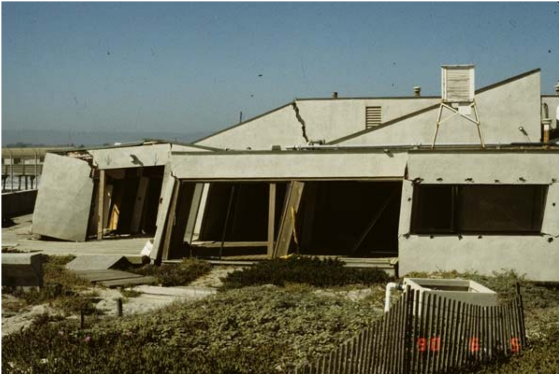
Figure 3-24. Photo of the Moss Landing Marine Laboratory facility, Monterey County, CA, destroyed as a result of about 1.2m of displacement due to liquefaction-induced lateral spreading caused by the M 6.9 1989 Loma Prieta earthquake. Ground motions at this site were sufficiently low that the structure would likely have survived the earthquake with minimal damage had the lateral spreading not occurred. Photograph by John Tinsley, U. S. Geological Survey.
