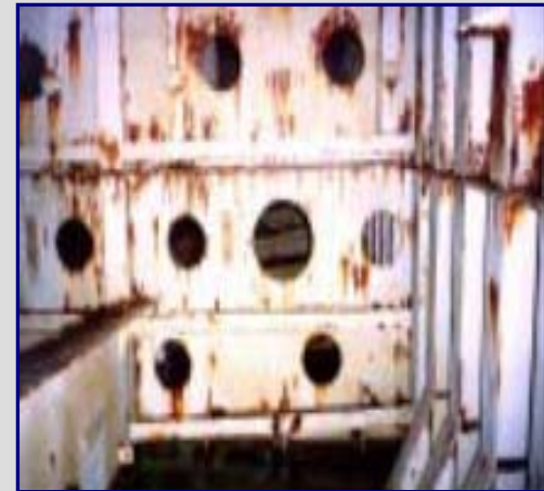
Corrosion is a common problem in shipboard tanks
