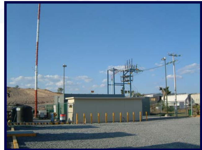
Mexican Landfill Biogas to Energy Plant
