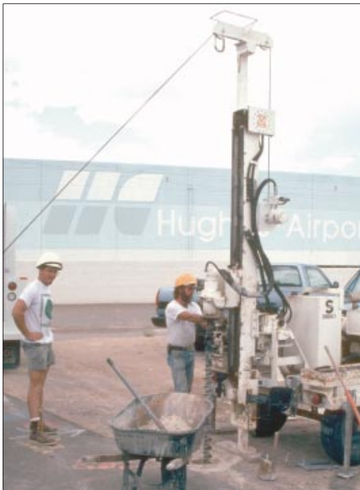
A shallow monitoring well being installed in the Las Vegas urban area, August 1993. Photograph by Kenneth J. Covay, U.S. Geological Survey.
