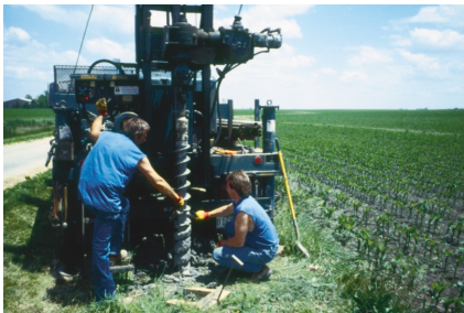
Figure 11. Study-Unit staff installed 57 wells to sample recently recharged ground water. Assistance and geological expertise was provided by the Illinois State Geological Survey. (Photograph by William S. Morrow, Jr., USGS.)
