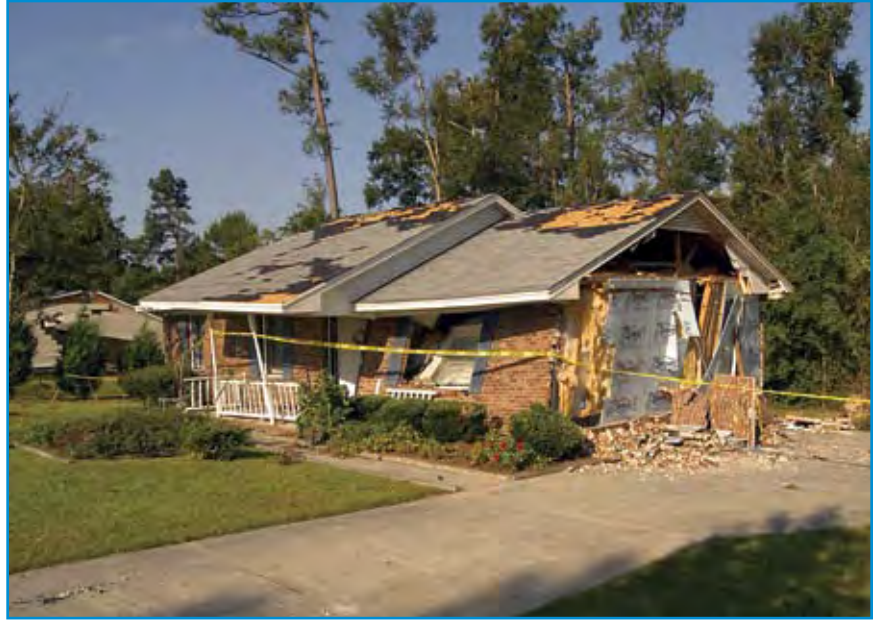
Hurricane Frances tornado damage, Sumter County, SC September 6, 2004/ Photo by Marvin Nauman/FEMA
