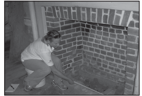
Lauren Noe, seasonal architectural technician, measures the stabilized basement fireplace at Rural Plains.
