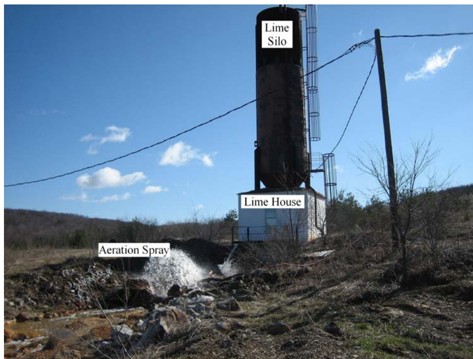
Figure 7-2. Photograph of the PBS Job #1 Lime House and Aeration Spray Source: Site Visit Report Pennsylvania Coal Mine Acid Drainage Treatment Systems (ERG, 2006)
