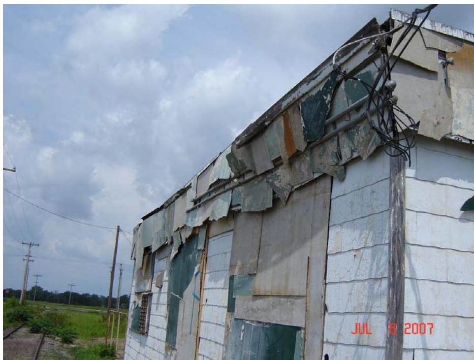
Building 235 with Additional Transite
