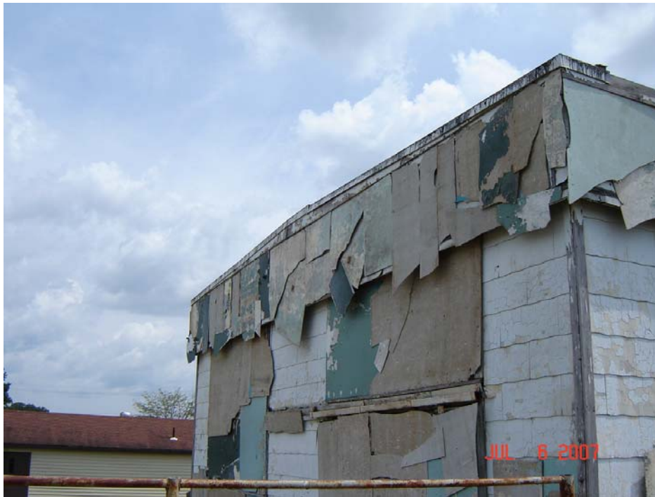
Building 235 with Additional Transite
