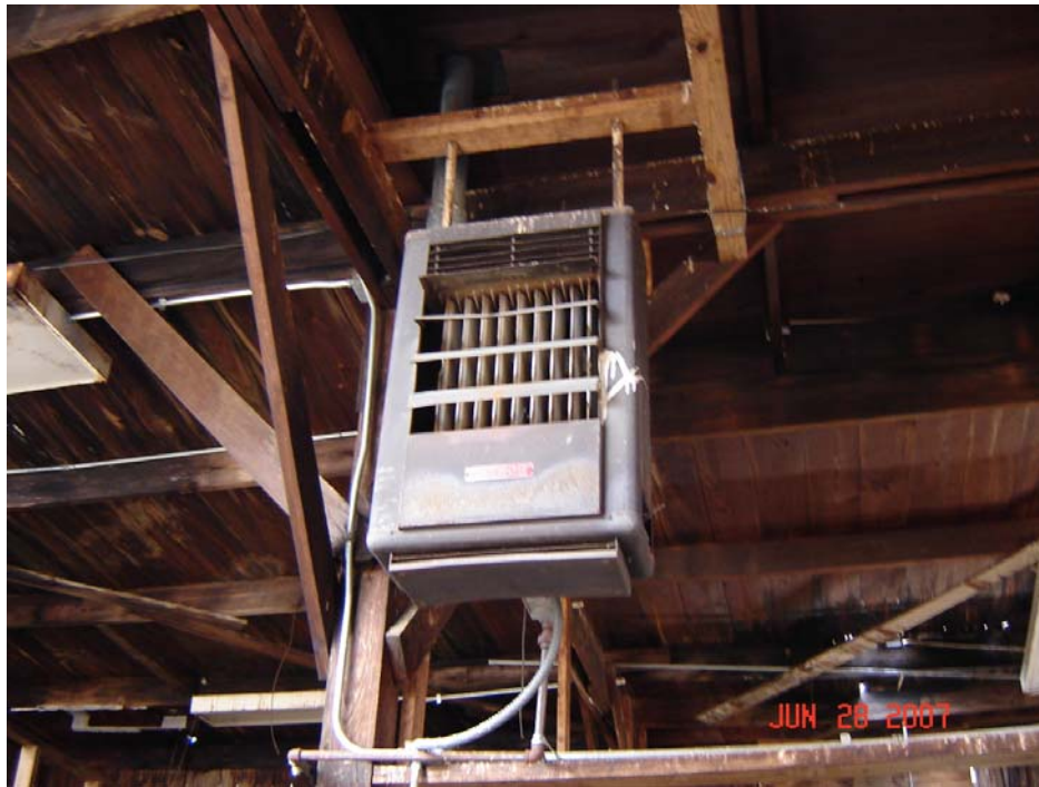
Gas Heater (No Asbestos-Containing Materials)
