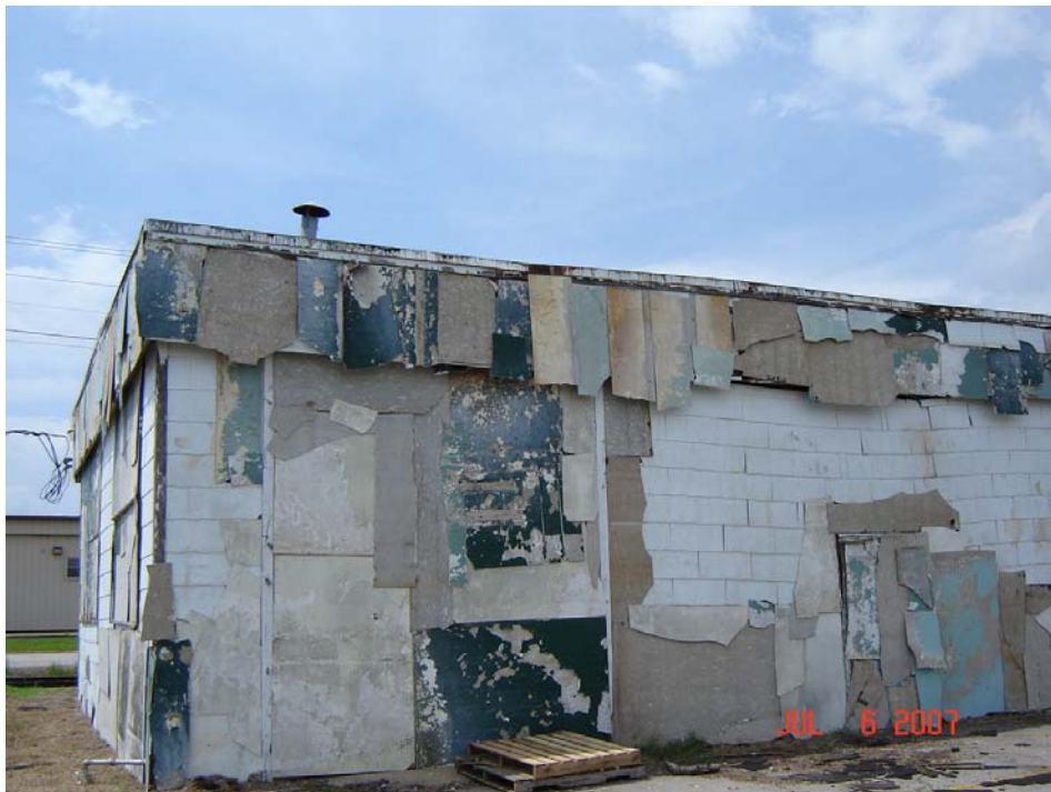
Building 235 with Additional Transite
