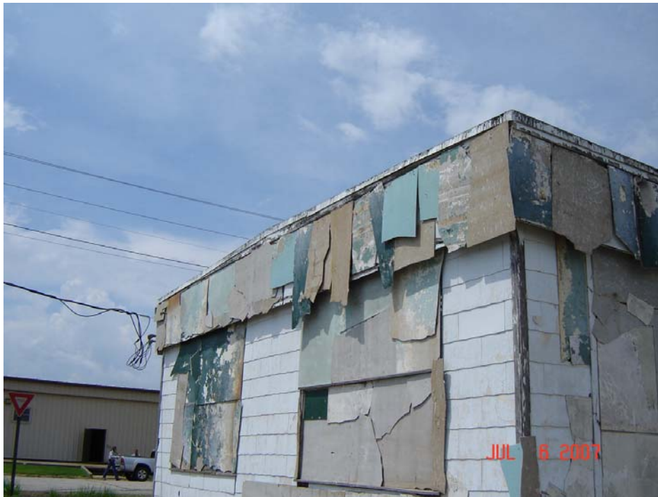
Building 235 with Additional Transite
