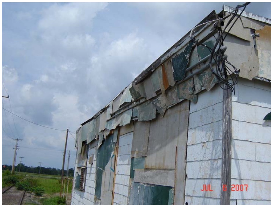
Building 235 with Additional Transite
