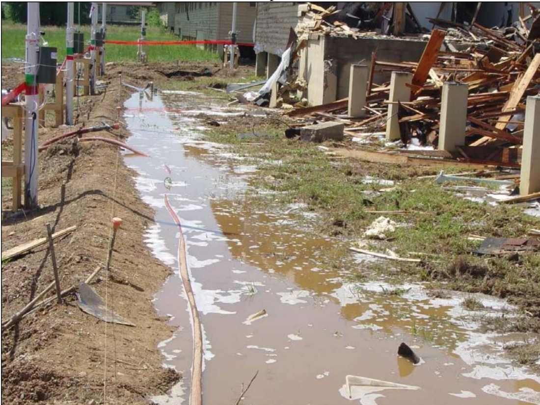
Figure 4-10. Water accumulation near the berm during the AACM demolition.
