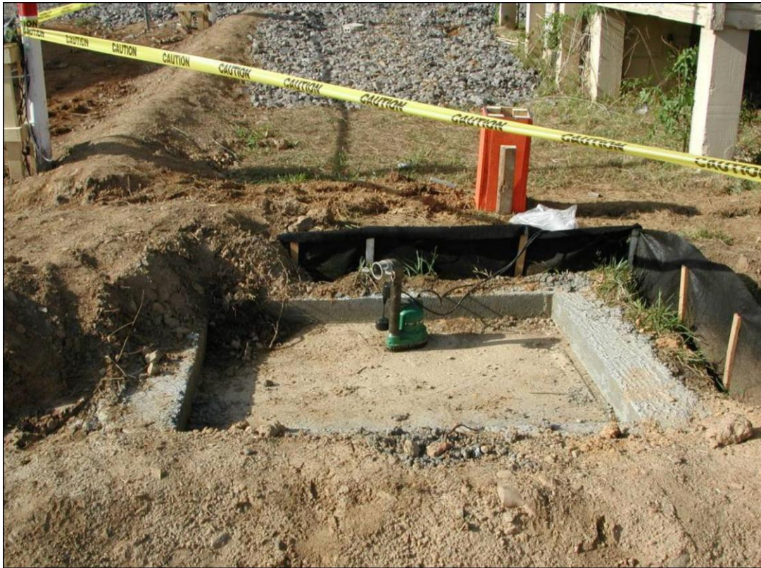
Figure 4-9. Pooled surface water collection sump.
