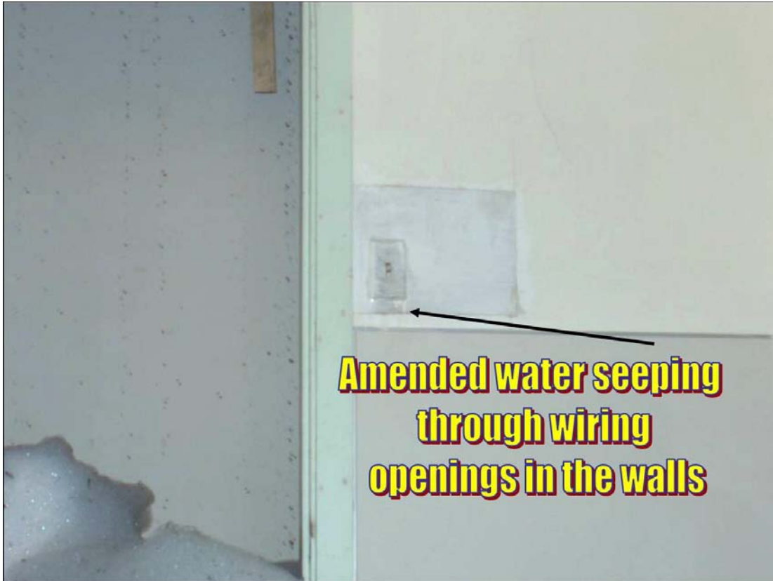
Figure 4-27. Amended Water seeping through wall openings.
