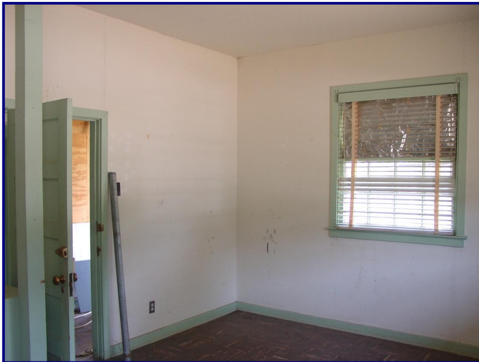
Figure 3-3. Interior view of Building #3602 (NESHAP). Interior finishes are gypsum wallboard (ceiling and walls) and nine-by-nine-inch resilient floor tile.
