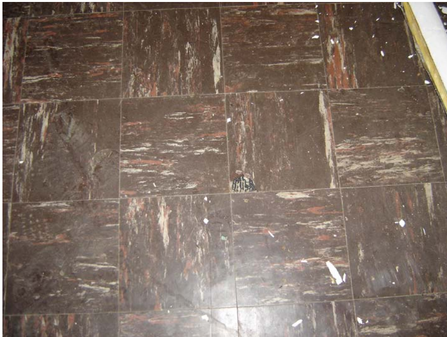
Asbestos Containing 9" x 9" Brown Floor Tile
