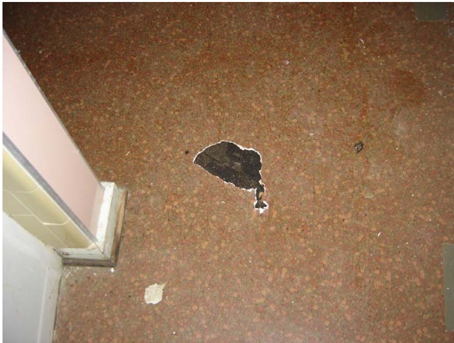
Asbestos Containing Multi-Colored Linoleum
