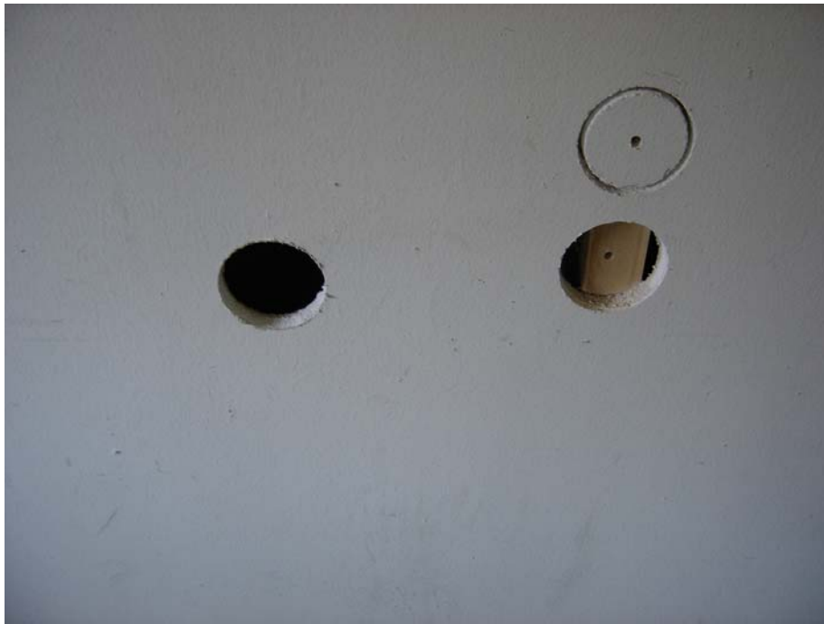
Asbestos Containing Drywall Joint Compound
