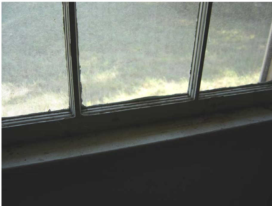
Asbestos Containing Window Glazing
