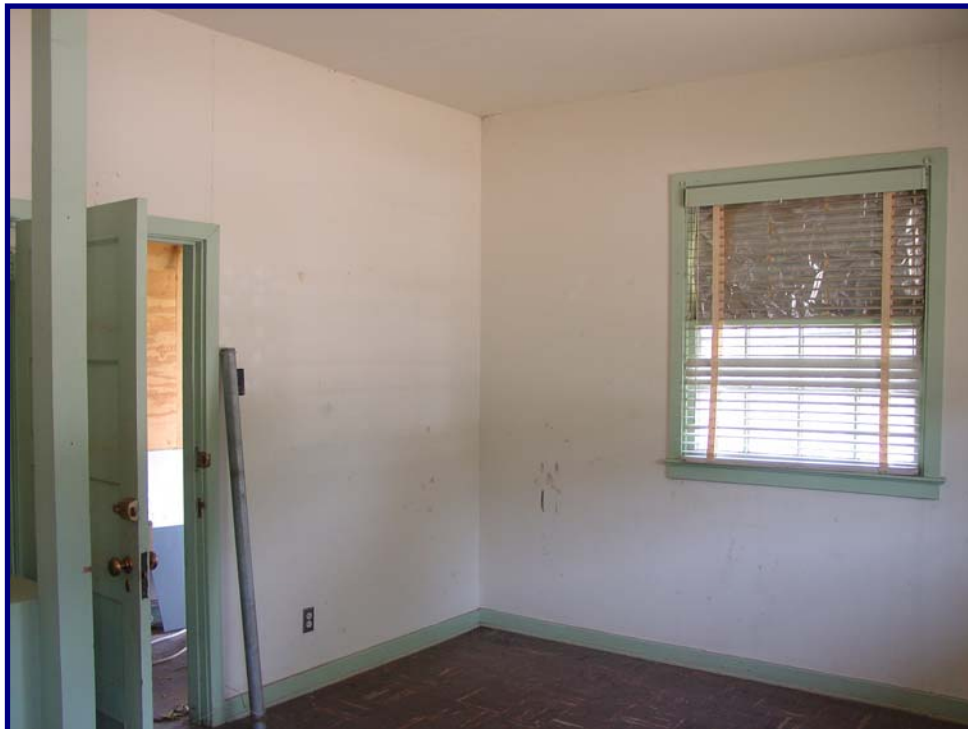
Figure A-4. Interior view of Building #3602. Interior finishes are gypsum wallboard (ceiling and walls) and 9- by 9-inch resilient floor tile.
