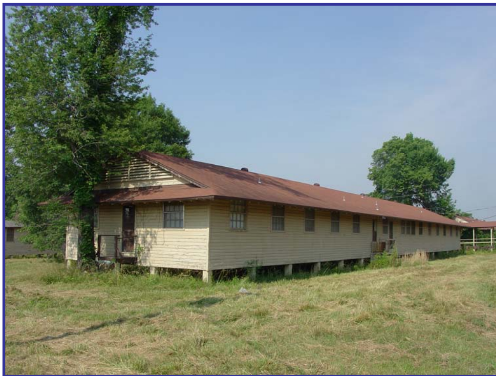
Figure A-3. (Top) Exterior view of Building #3602 (NESHAP Method) and (Bottom) #3607 (Alternative Method). Dimensions: 30-feet by 150-feet.
