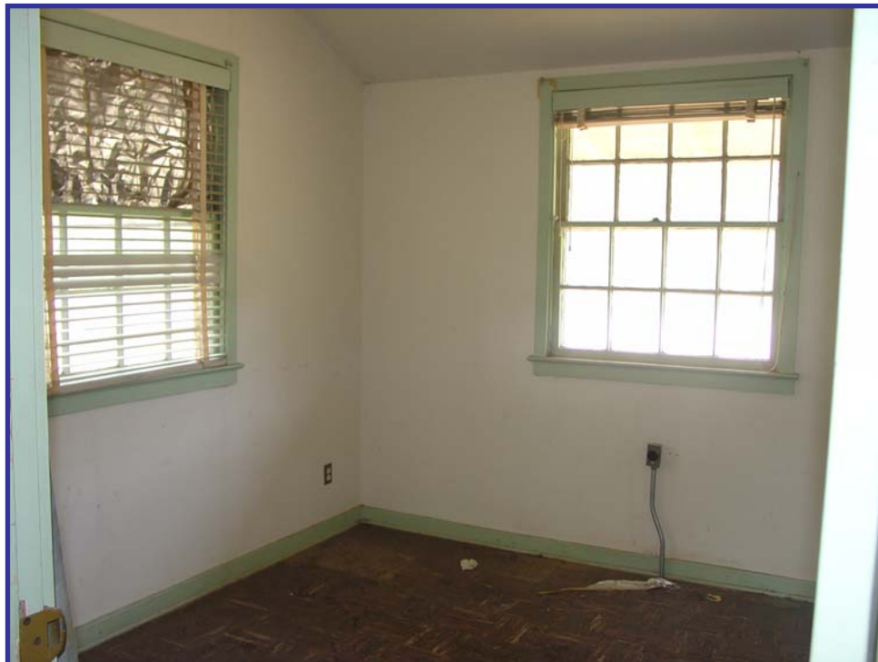
Figure A-5. Interior view of Building #3607. Interior finishes are gypsum wallboard (ceiling and walls) and 9- by 9-inch resilient floor tile.
