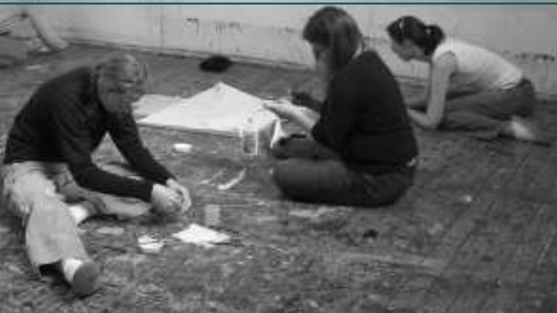
During renovation work on the Pollock-Krasner House and Study Center, Jackson Pollock's studio floor was protected by a layer of foam board and a tarpaulin to prevent damage to the fragile paint surface.
