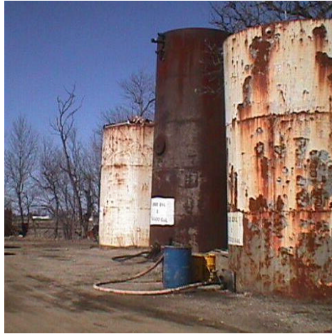
Single-wall tank directly on soil and without spill control
