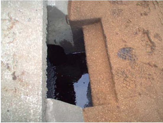
Fig. 7 – Rainwater sewer inlet.
